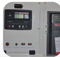
Control Panel & MCB
